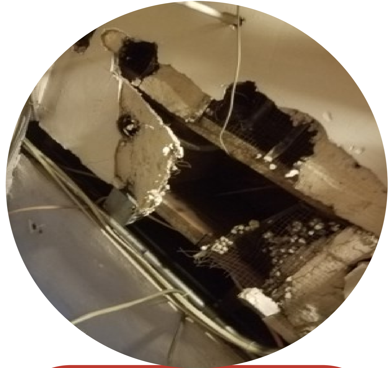
Crumbling building features
