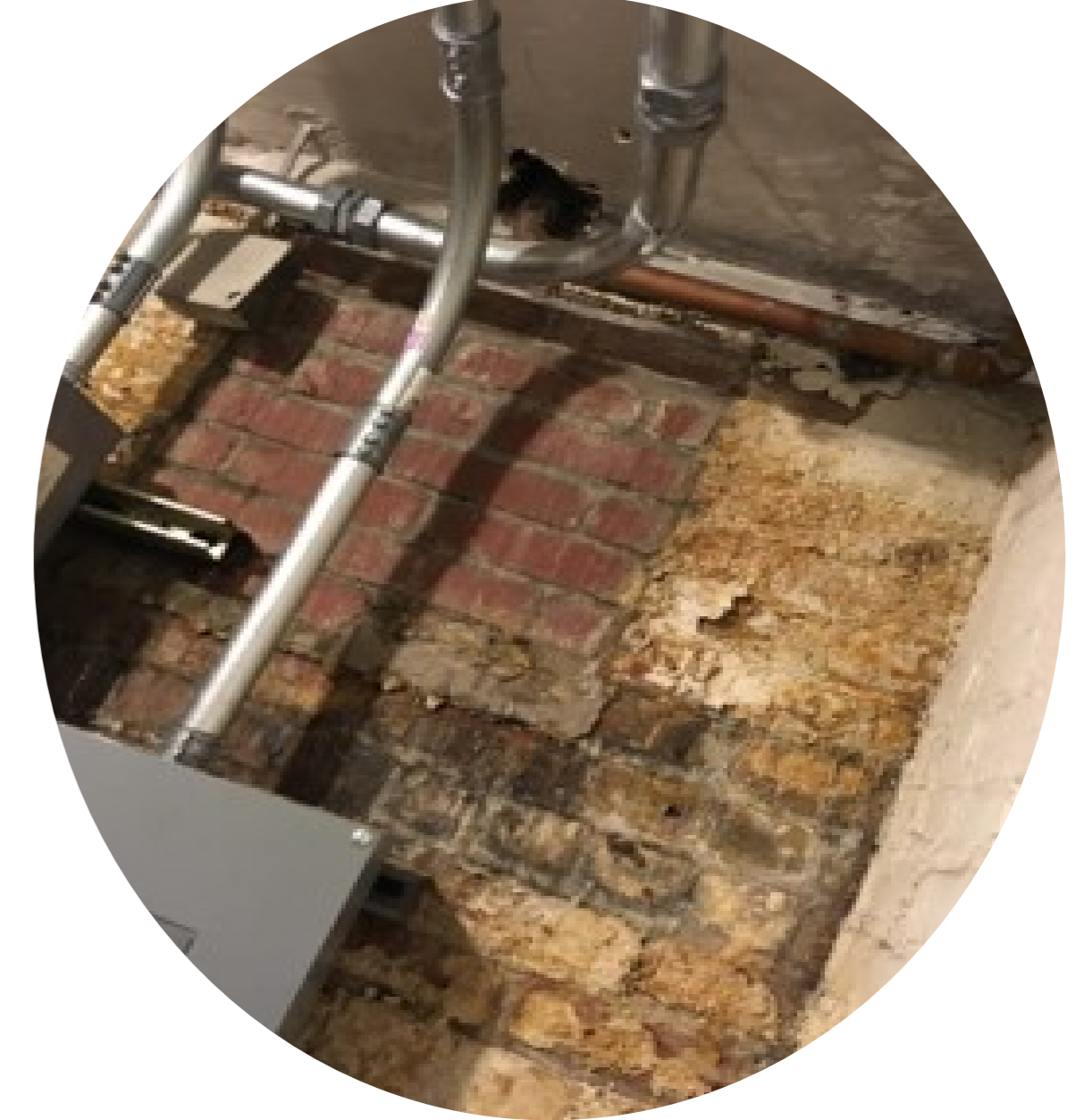
Vulnerable electrical systems
