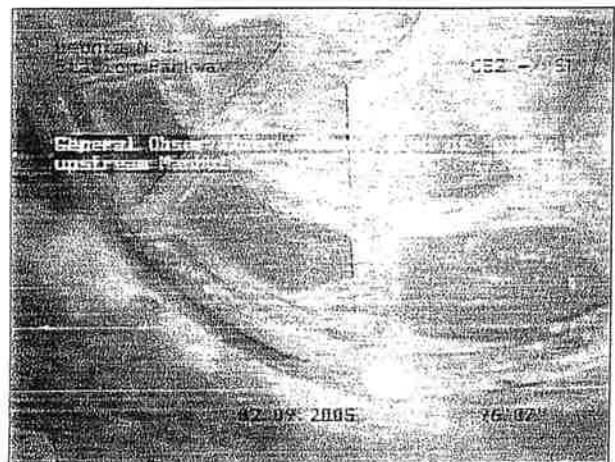
Photo: 38a, Tape/Media No.: 1[TV30], 00:59:44 96.6FT, General Observation, Remark: End of Survey upstream Manhole
